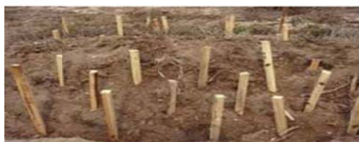
each layer of branches is followed by a layer of compacted soil.
